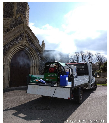
Diesel Particulates from boiler.
